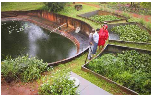
Fig .12.7 (a) DEWATS system at Auroville
