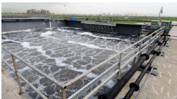
Figure 22.4 A view of sewage treatment plant
